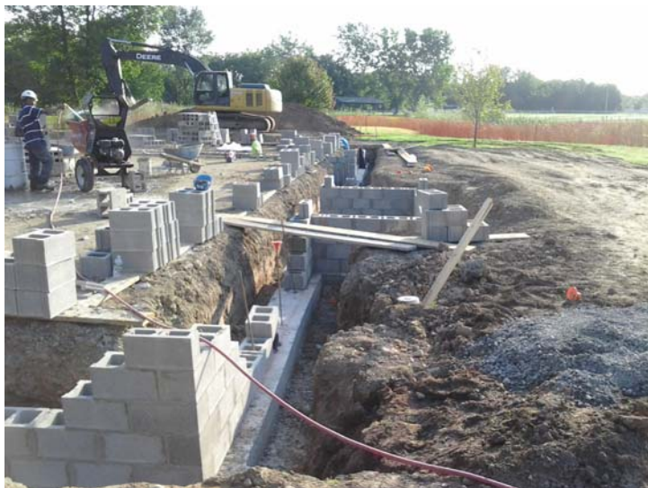
Pictured above is the foundation for the new Lodge at Sweden Town Park, Redman Road.
